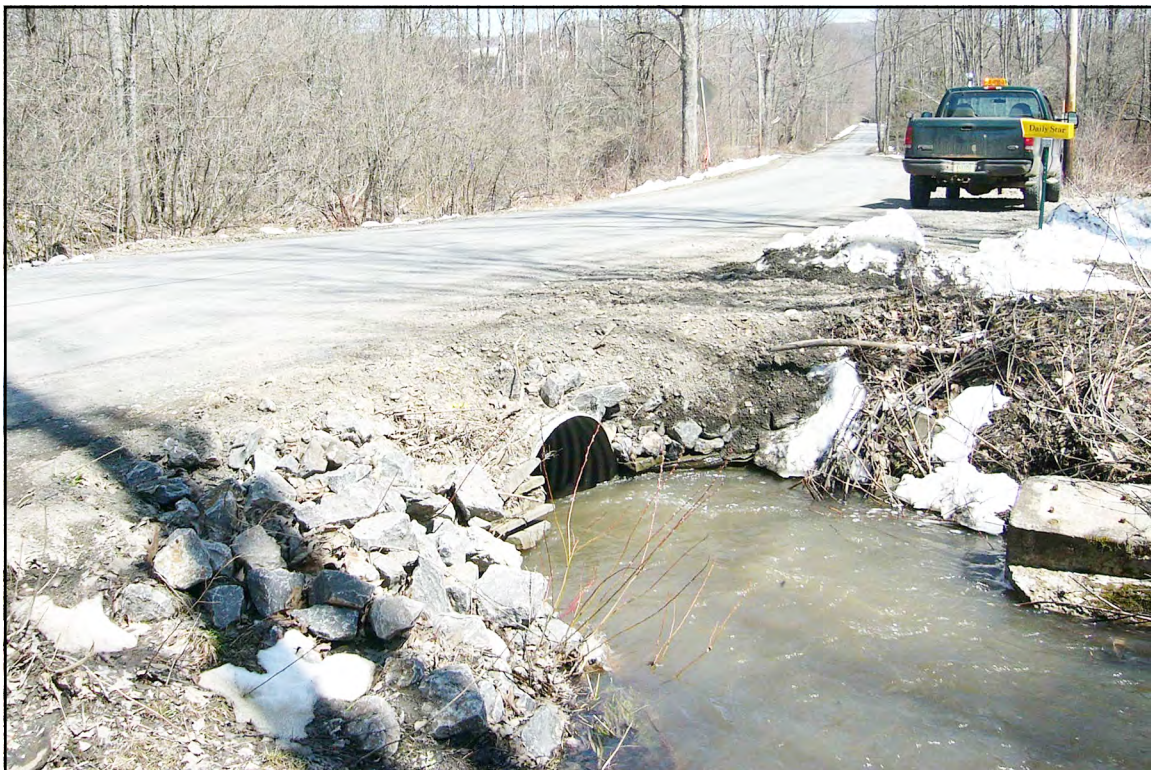
Roadway grade elevation increased, but culvert not changed
