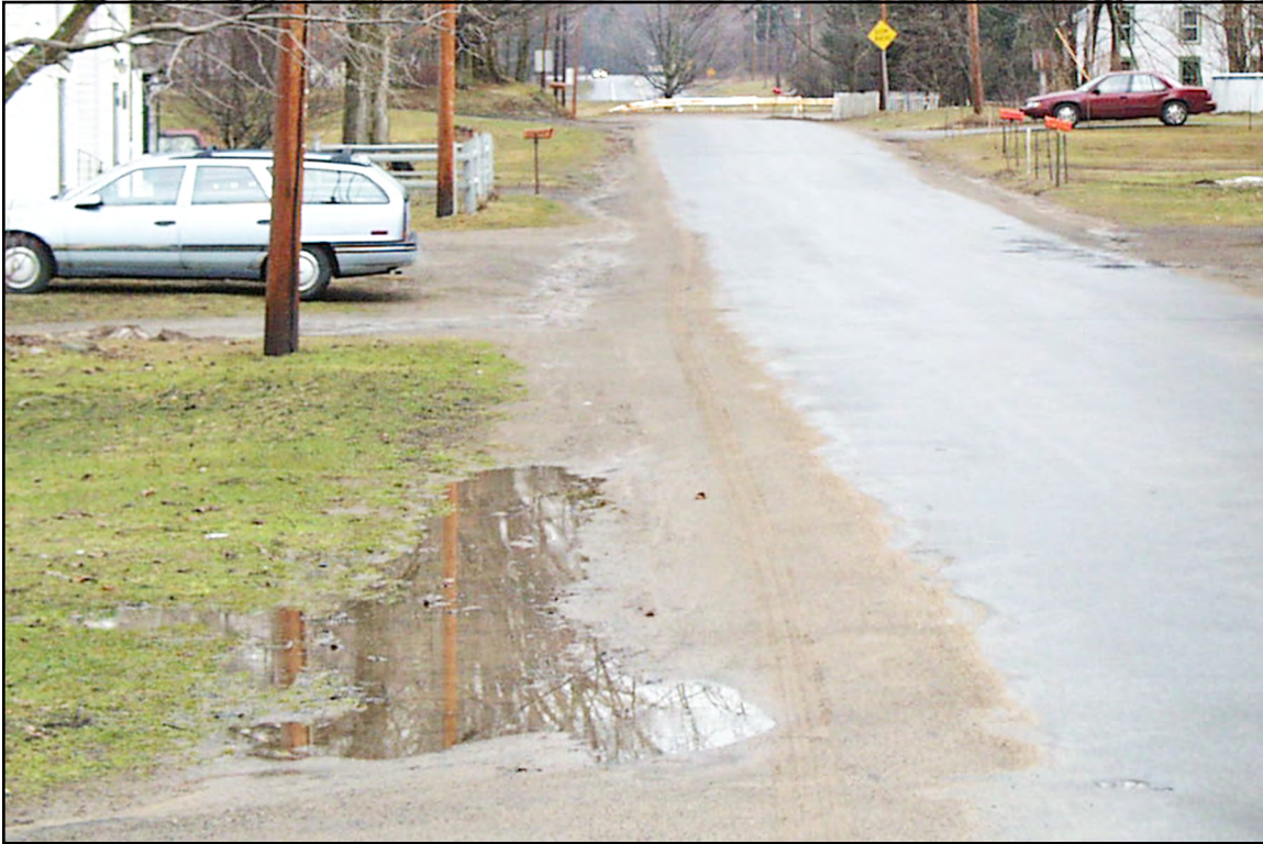
Raised street elevation causing flooding or retention of runoff
