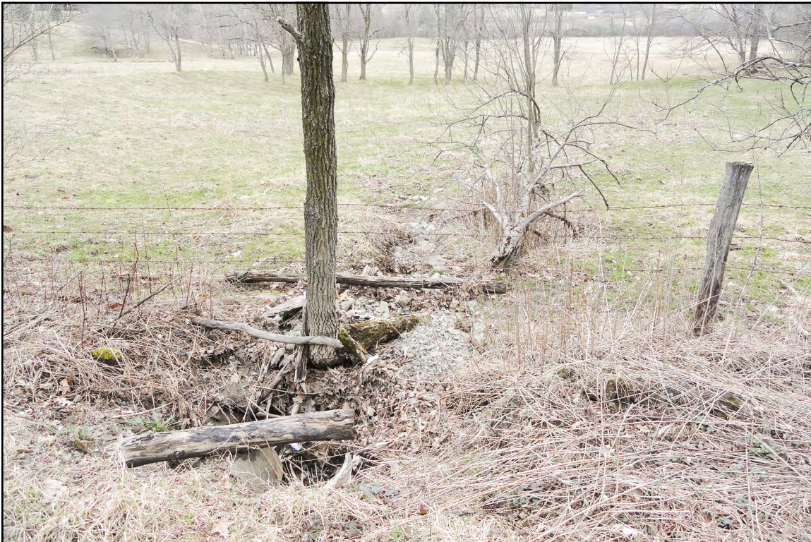
Unmaintained drainage ditch
