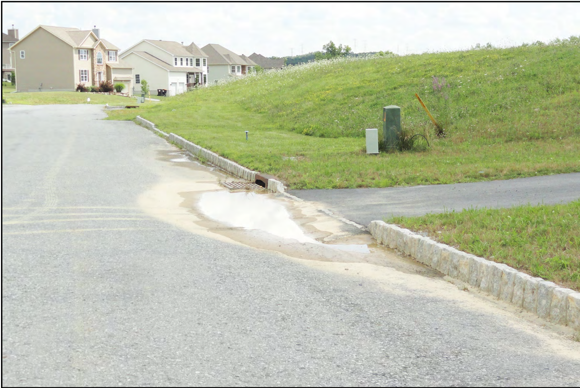
Discharge from higher driveway pouring onto road
