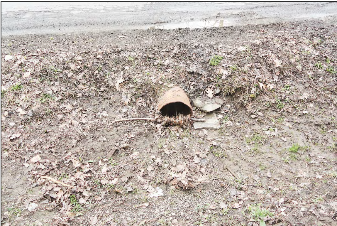
Drainage pipe in need of cleaning
